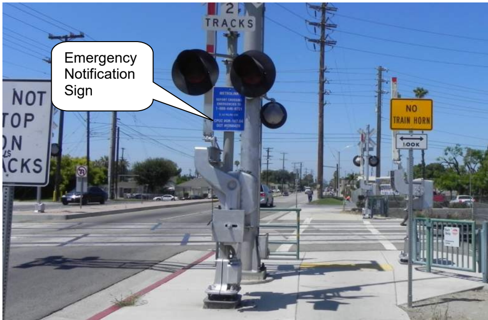
Figure 3-18. Emergency Notification Sign Placement
