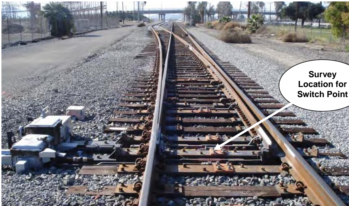
Photograph of Switch
